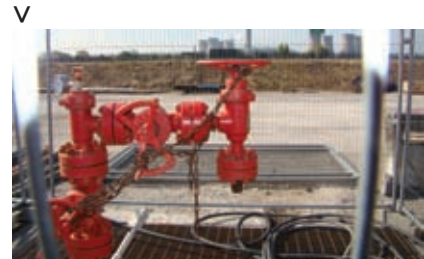
Well head at DG1
