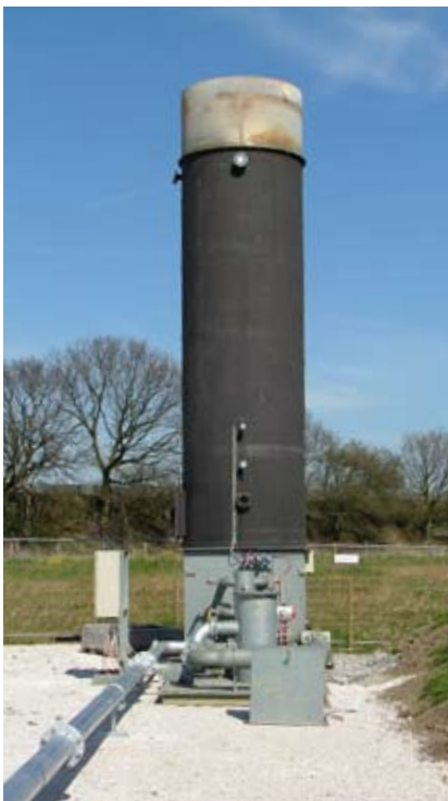
< Shrouded flare used for monitoring production test at Doe Green site in Cheshire
